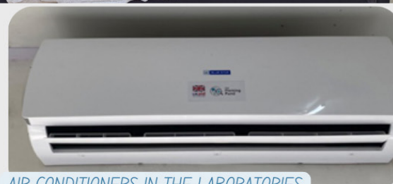
AIR CONDITIONERS IN THE LABORATORIES
